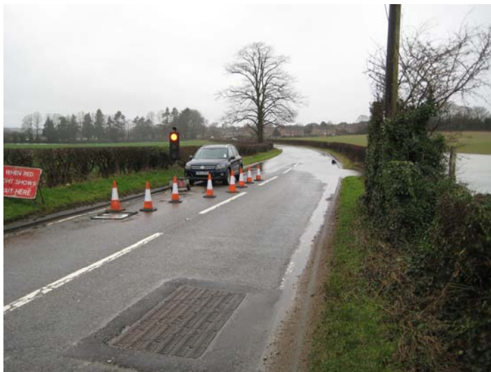
Figure 2: Flooding Long Lane near High Field Road 200mm deep surface water
